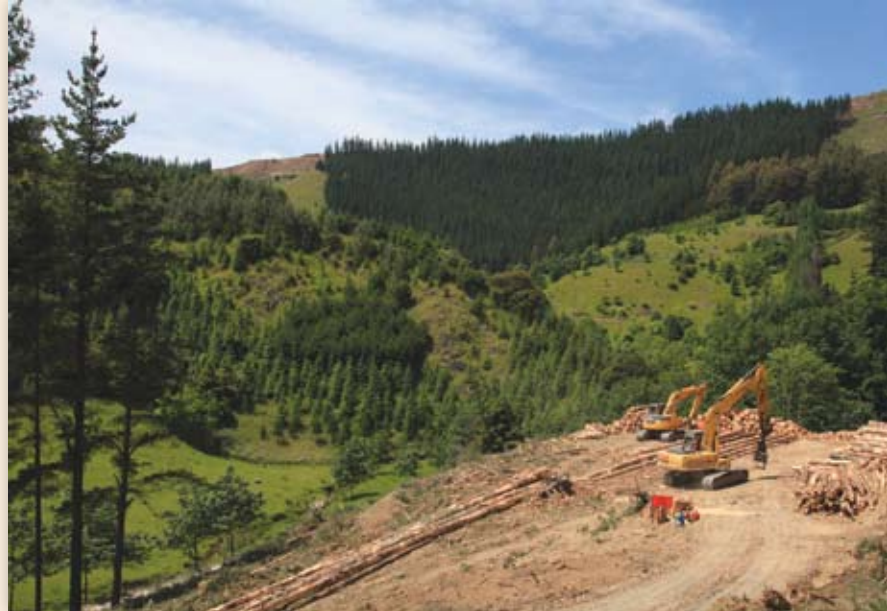
0.6 ha valley skid site and the 4 ha ridge-top logging in the background.
